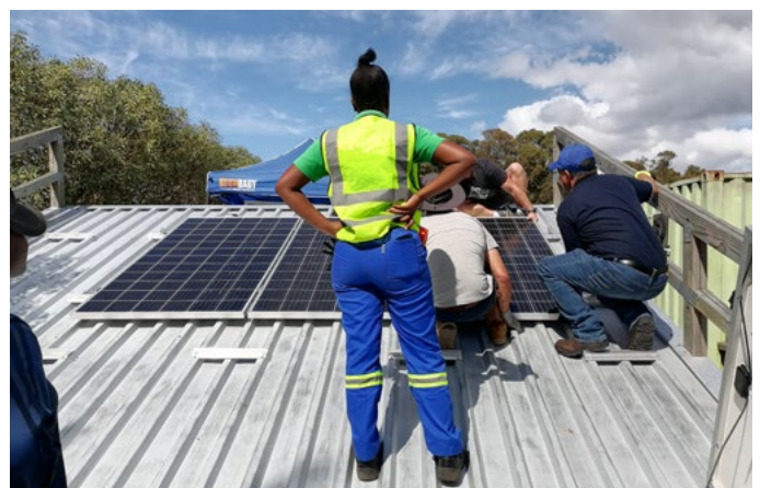
Understand commissioning of a PV system
